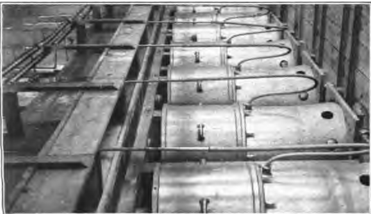
C. SUCTION FILTERS IN NEW PLANT, SHOWING LEACHING POTS ABOVE.
